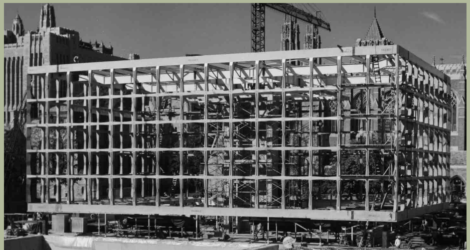
The Beinecke Rare Book and Manuscript Library, shown during construction in 1961–1963, is one of relatively few campus buildings for which a maintenance endowment has been created (the gift of members of the Beinecke family).
